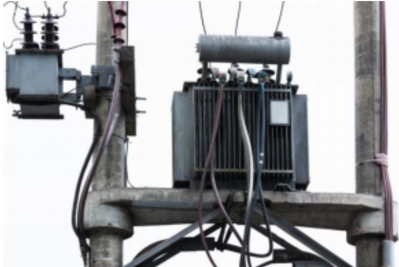
FIG:8, DISTRIBUTION TRANSFORMER
