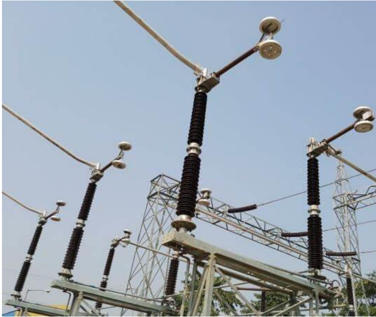
Electrical Isolation Switch
