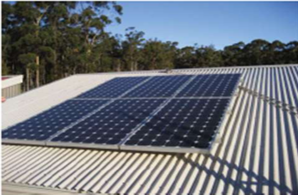
Figure 4.22 Even this small shadow can reduce the amount of electricity a module produces – a small shaded area can, under certain circumstances reduce module output by 80–90 per cent as well as affecting the rest of the array
